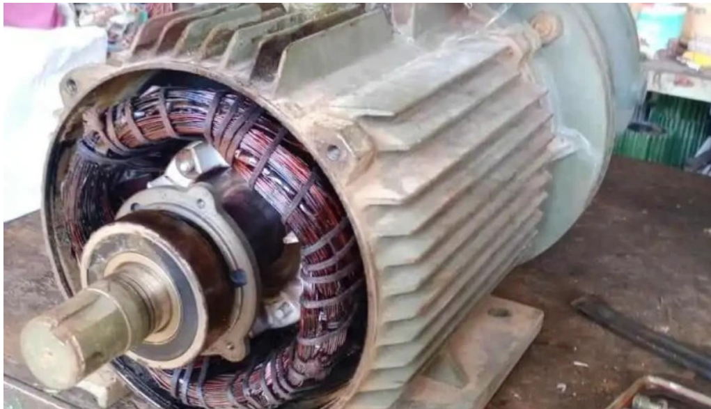
Electromecanica nessier interior
